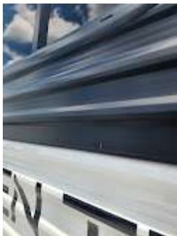
line 1 damaged metal.jpeg 851K
