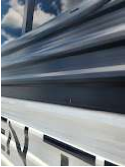
line 1 damaged metal 2.jpeg 851K
