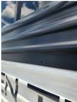
line 1 damaged metal 2.jpeg 851K
