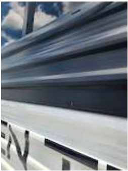
line 1 damaged metal.jpeg 851K
